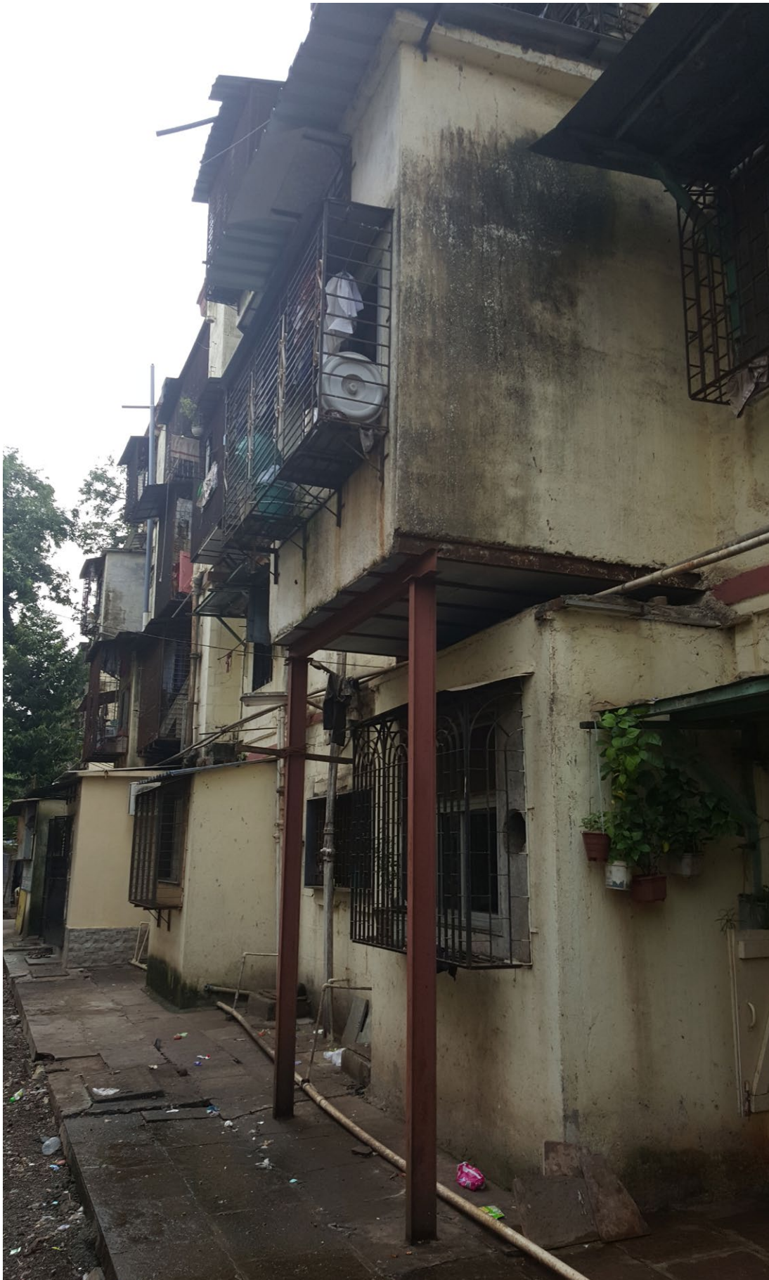
One of the 42 buildings at BDD chawl. Some of the residents have created more space for themselves by extending their home using steel beams.
