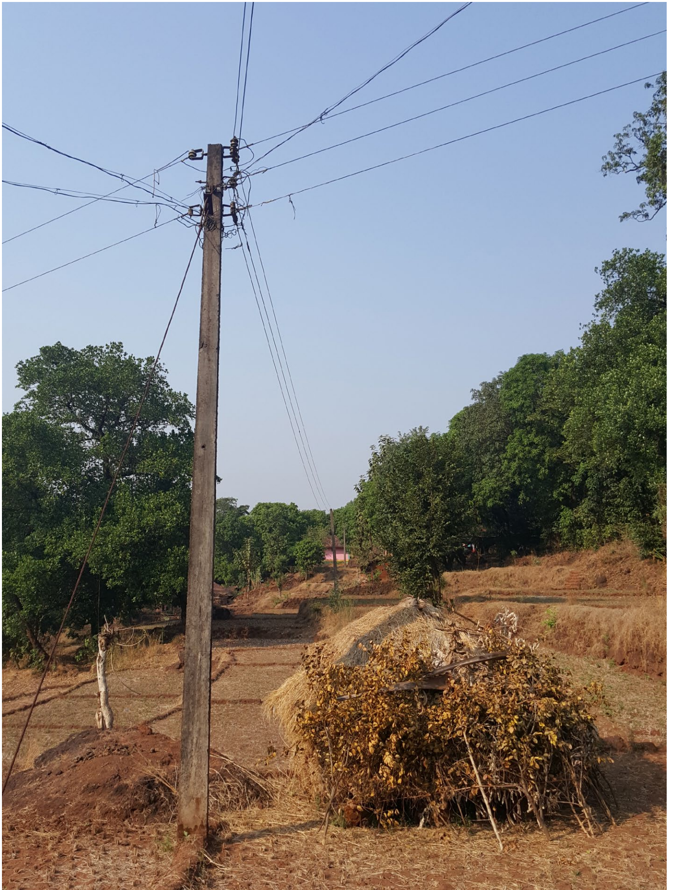
Electrical pole in Songiri. Few of the villagers have landline phones. Most of them use mobile phones. Songiri only receives reception from one phone company.
